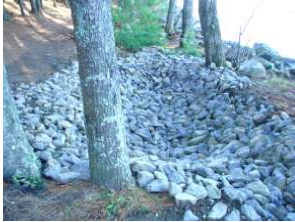
Rocked drainage diversion and plunge-pool to capture stormwater and any eroded road material from hill #2, 12, 15
